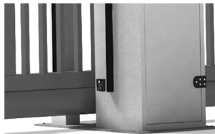
Control cabinet with photocell.
